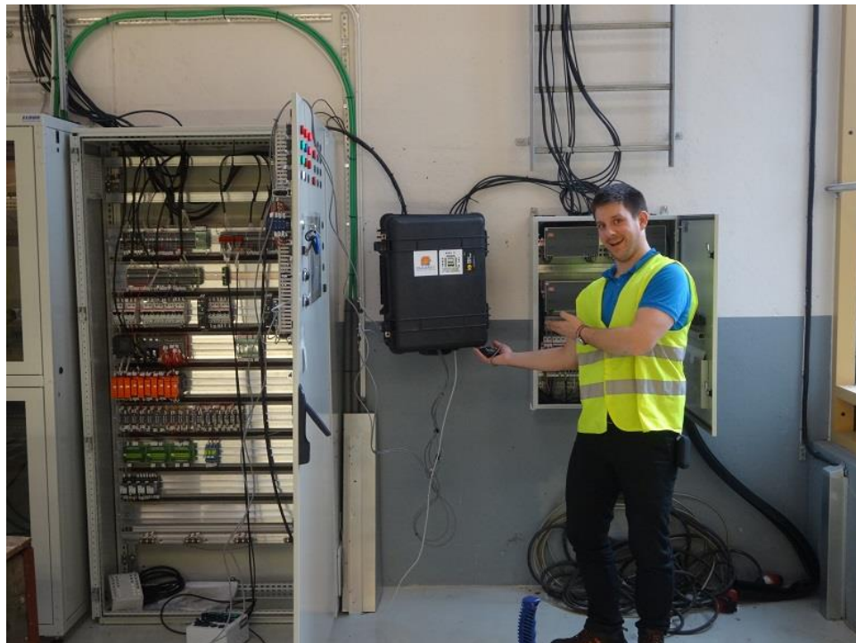
Platform screen doors controller installed in Stockholm (Citybanan)
